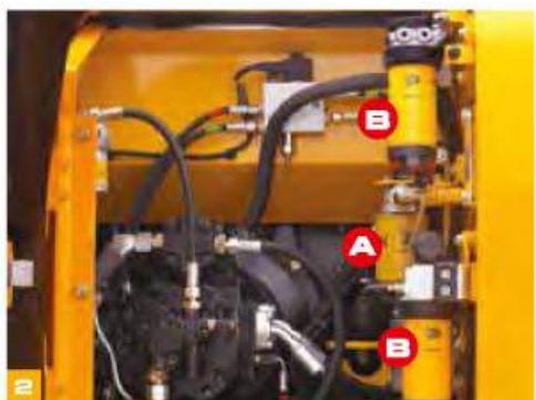
(A) Hydraulics oil filters (B) Fuel filters
